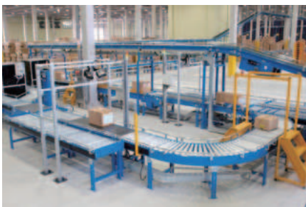
13. Company A MHE Conveyor System
