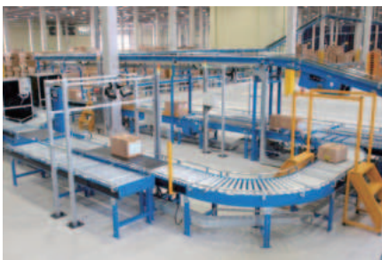
13. A사 MHE Conveyor System
